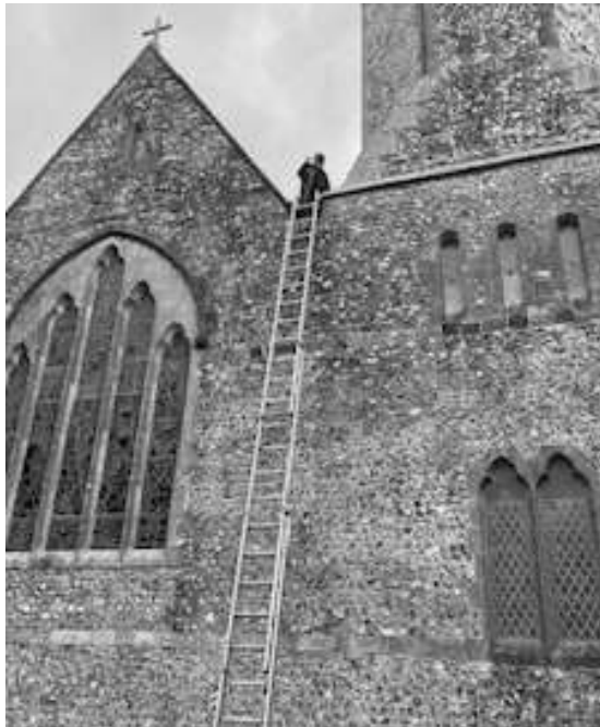
Picture by Rob Hollis who says 'Eric the Church repair man checking gutters and roof'.
